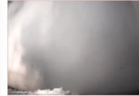
Novec 1230 discharge [TR + 00:00:58]
